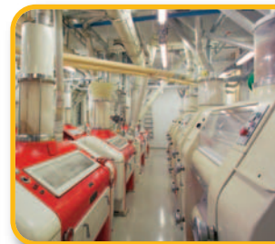
Appropriately protected equipment at a UK grain mill
